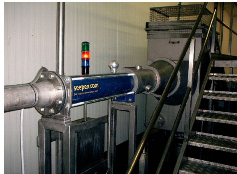
seepex BTM pump with integral stone trap and cutting knives handles waste vegetables, replacing both widethroat pump with grinder and the screw conveyor
